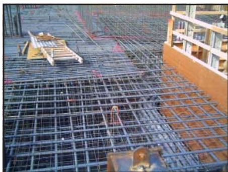
75 ksi rebar in place of conventional 650 ksi bar in the foundation of downtown Seattle's Cosmopolitan Tower
