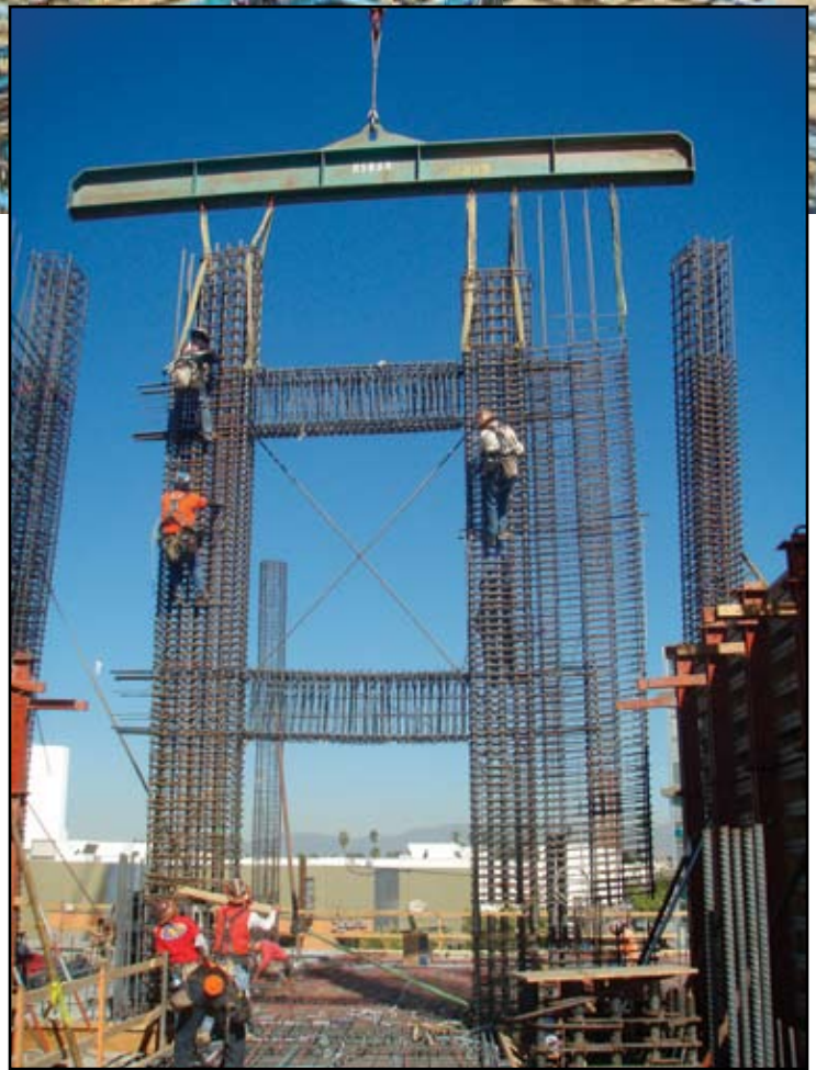
Shear wall rebar was detailed to allow pre-tying of cages offsite. This minimized field labor and accelerated construction.
