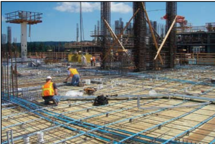
Slabs are typically 8-inch thick with a combination of post-tensioning and mild rebar. Note that exhaust ducts were buried in the slabs, along with most electrical conduit.
