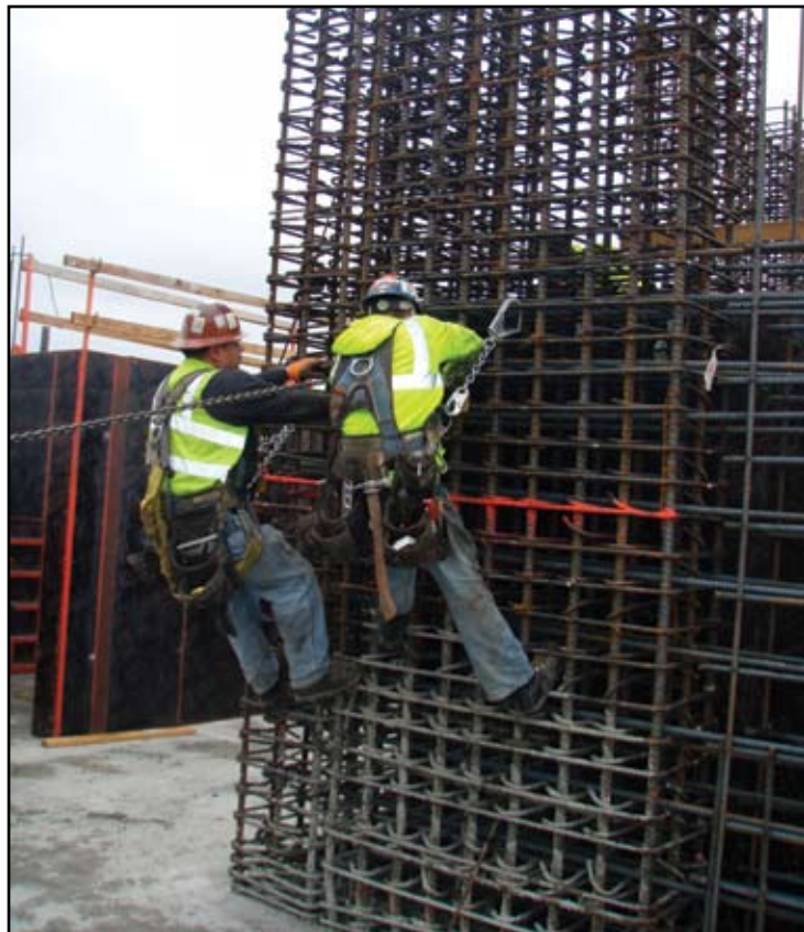
Rebar ties with a 90 ksi yield strength substantially reduced congestion at columns and shear wall boundaries.
