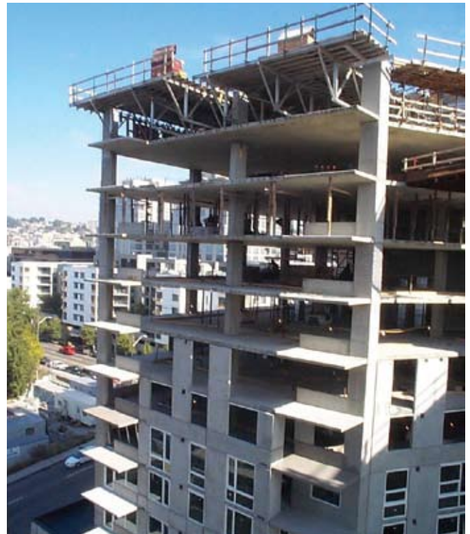
Conventional flying form trusses immediately after flying. Reshores will be installed prior to placing the slab
