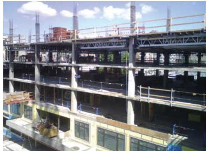
Column-hung flying deck forms prior to placing the slab. All slab loads are carried directly by the columns, resulting in open decks below the forms with no shores or reshores. This allows workers to move about freely
